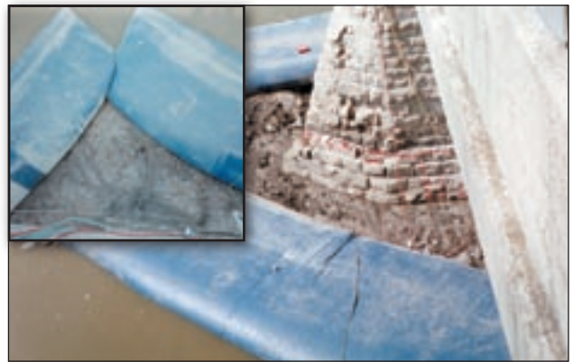
Maumee River, Miami, OH. Bridge Repair 200 linear feet of 6-ft barriers installed in 5 hours around individual bridge piers.
