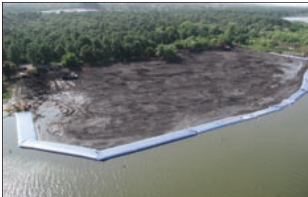
Dredging Project Lake Seminole, FL 1,500 linear feet of 5-, 6- and 7-ft barriers installed in 10 hours.
