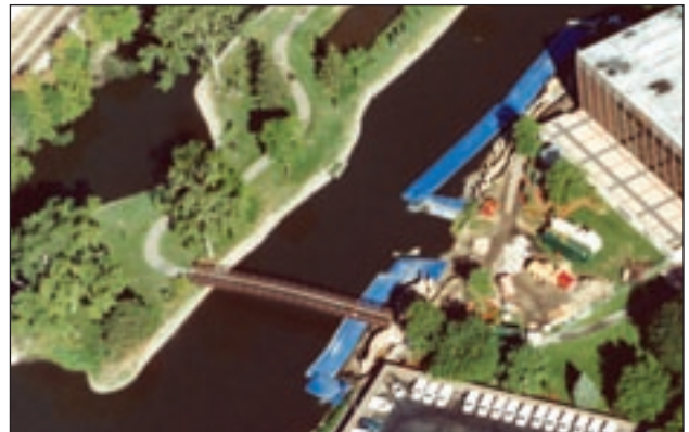
Shoreline Enhancement Elgin, IL Fox River 300 linear feet of 7-ft barriers installed in 7 hours.
