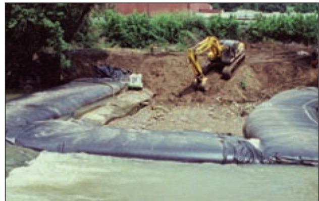
Roanoke River, Roanoke, VA Sewer Line Installation 250 linear feet of 6-ft barriers installed in 11 hours.
