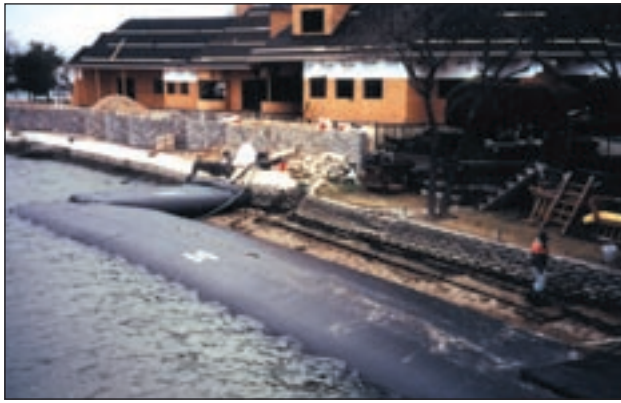
Eagle Lake, TX. Retaining Wall Repair 150 linear feet of 5-ft barriers installed in 3 hours.
