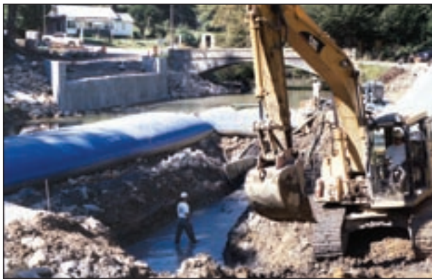
Middlefork River, Queens, WV Bridge Repair 150 linear feet of 5-ft barriers installed in 4 hours.
