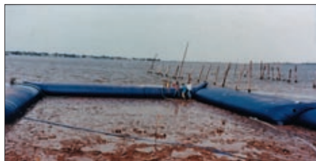
Wichita Falls, TX. Boat Ramp Installation 375 linear feet of 5-ft barriers installed in 5.5 hours.
