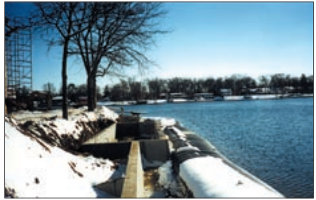
Elkhart, IN. Sea Wall Repair 350 linear feet of 3-ft barriers installed in 3 hours.
